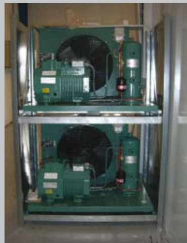
Redundant compressor system for cold store room -25°C
